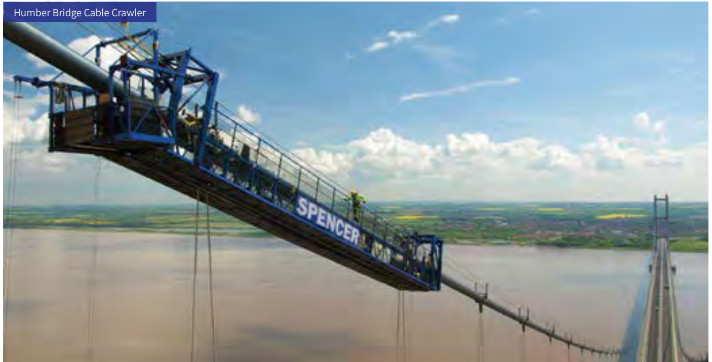
Humber Bridge Hanger Gantry
